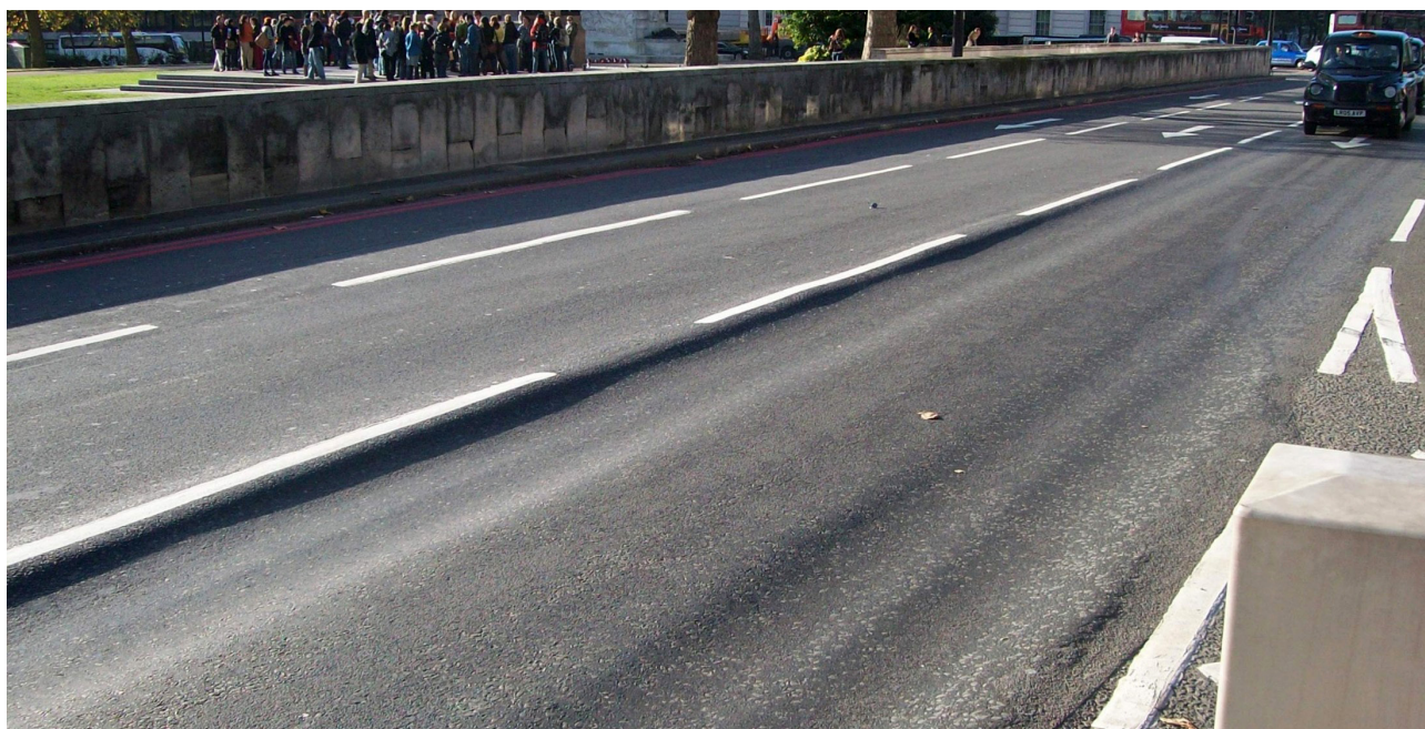
Figure 1: Example of permanent deformation
